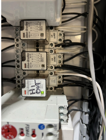
Vacuum pump / Condensate return controls
