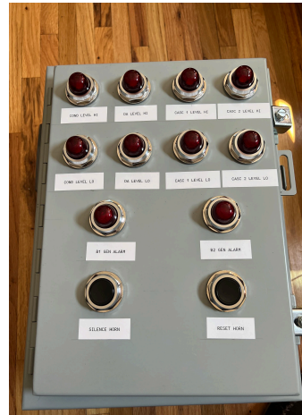
Remote alarm annunciator panels
