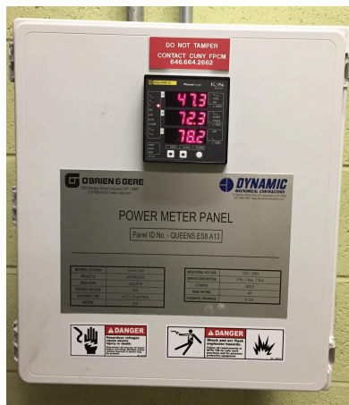
Electric power meter interface...
