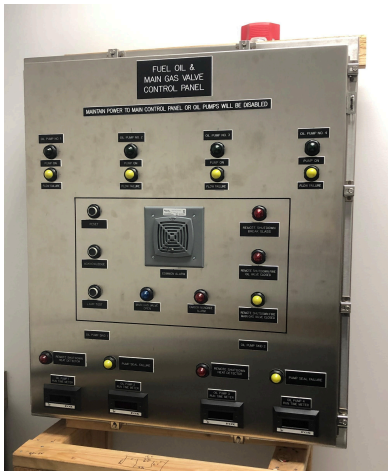
Fuel system controls
