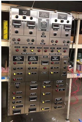
Balance of Plant controls
